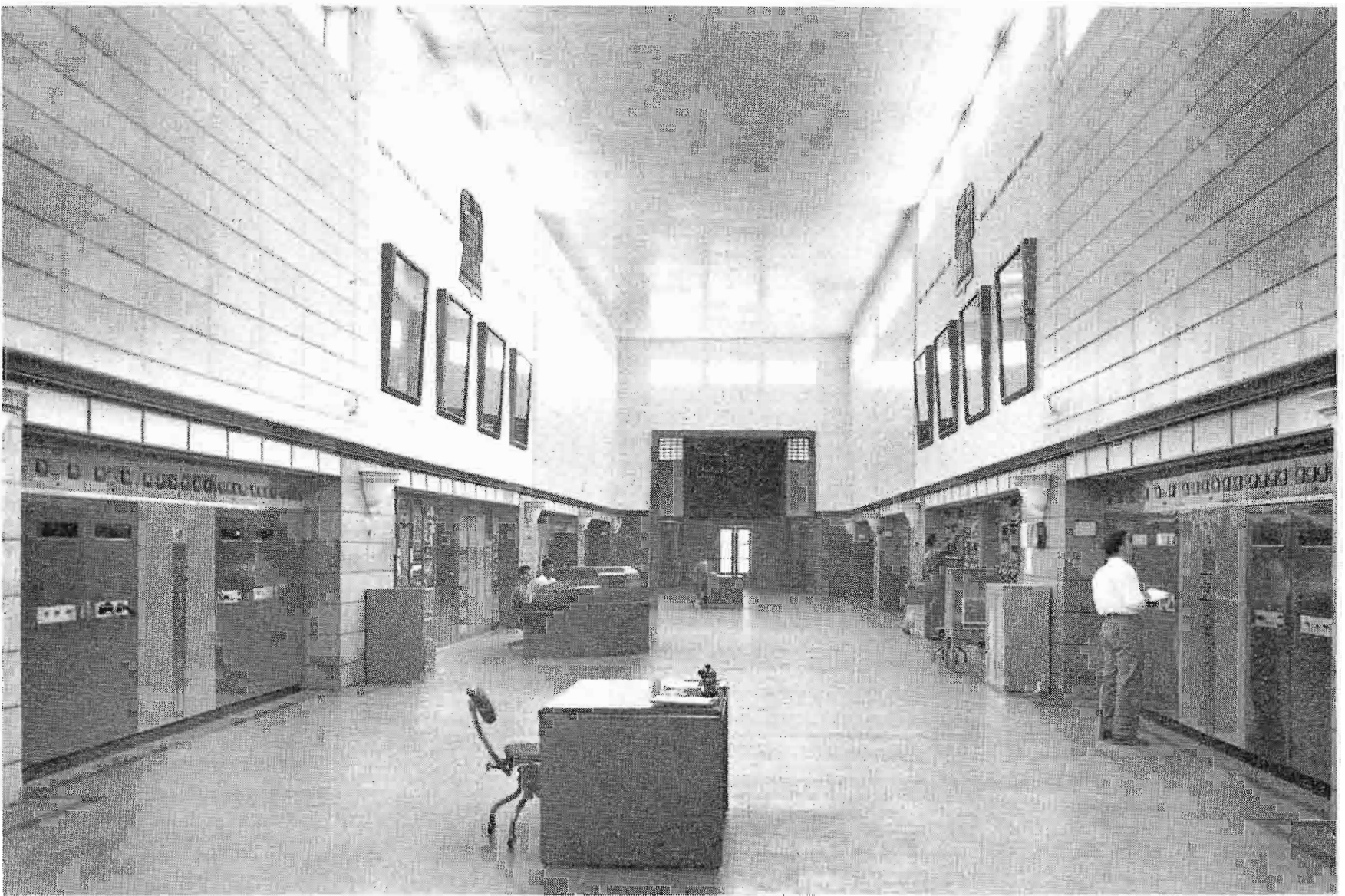
FIG. 39. Main transmitter hall at Gloria showing installation of eight RCA 50-KW Transmitters—four on each side.
