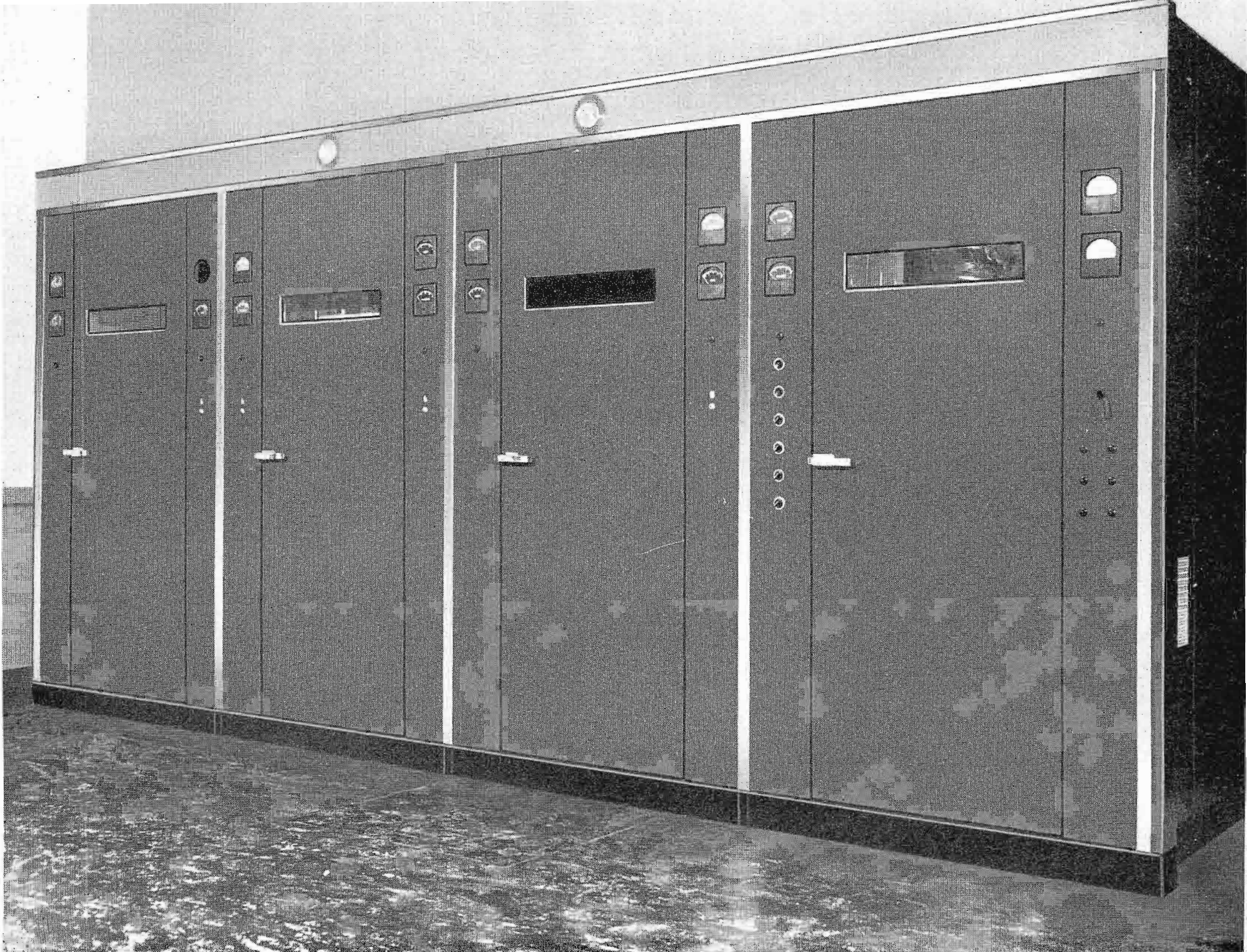
FIG. 1. Front view of RCA "Ampliphase" 50-KW AM Transmitter.
